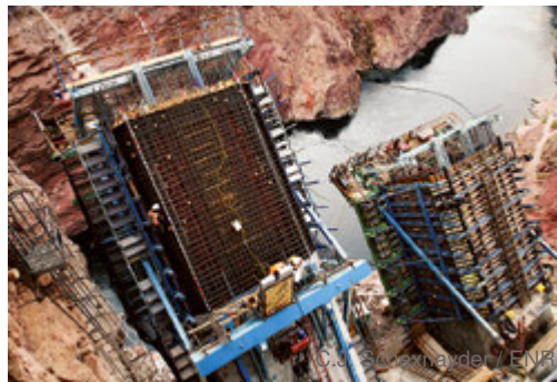
Once it has been vetted, a replacement cableway system will place girders and deck sections for the Hoover Dam bypass.
