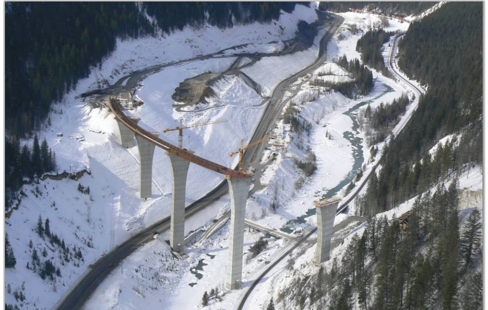
the first set of girders reaches the fourth and tallest pier in February 2007
