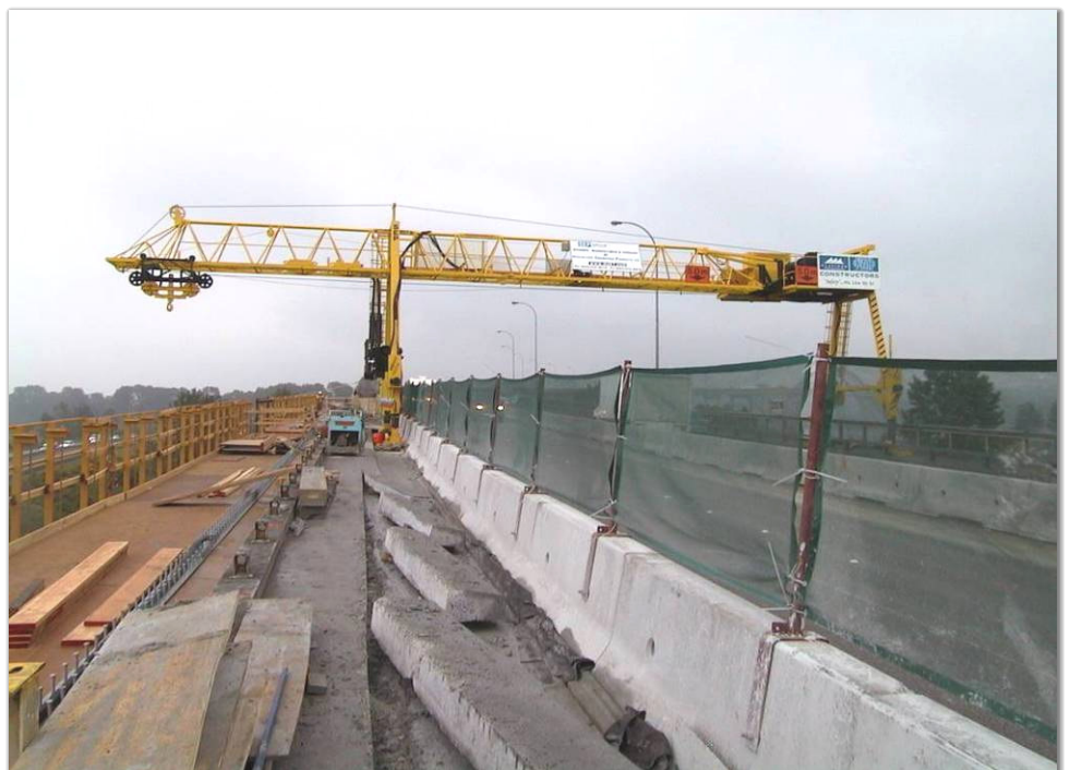
the rolling gantry crane that was employed had the capacity to pick loads from the ground
