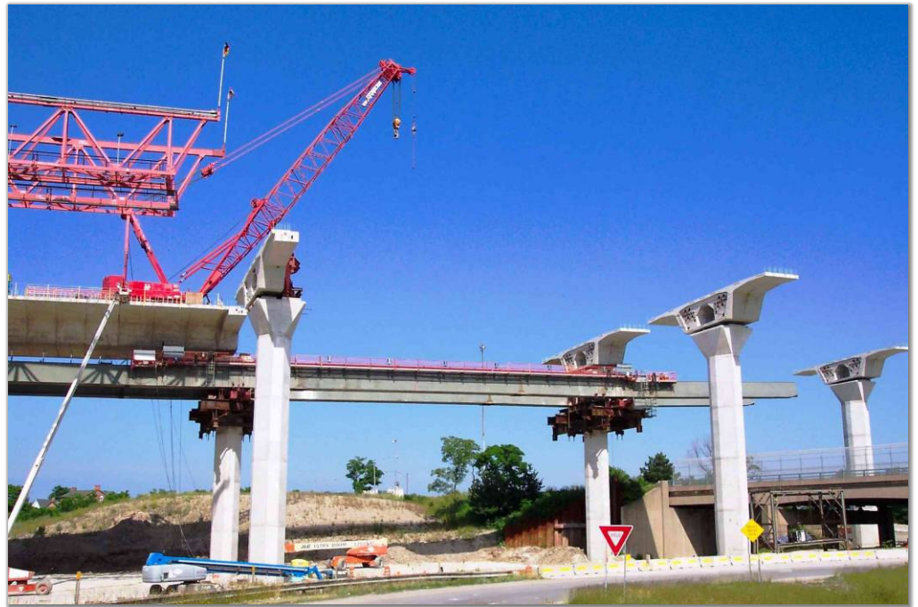
Under-slung launching girders are supported on suspended pier brackets over a maximum span of 50 metres
