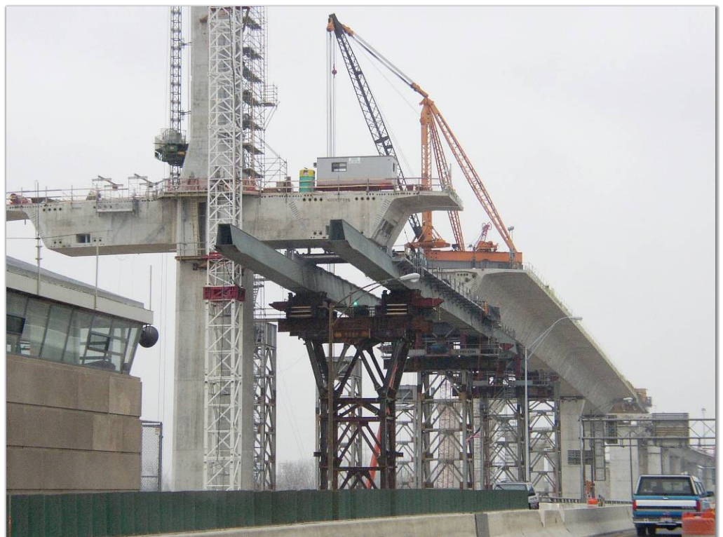
Launching girders supported on shoring towers in the river. A traveling derrick erected the precast concrete segments
