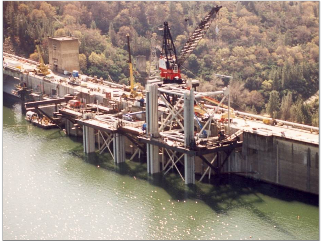
The massive temperature control device towers were lowered as each section was erected
